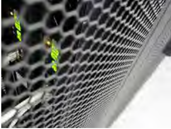
A New York City municipal data center. Photo by the NYC Department of Information Technology and Telecommunication , CC BY-NC-SA 2.0.
